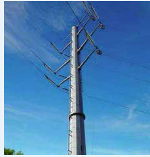
Power distribution poles
