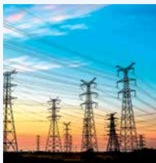
Power transmission tower
