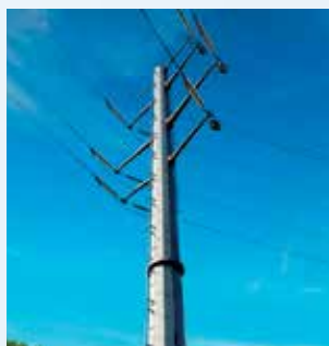
Power distribution poles
