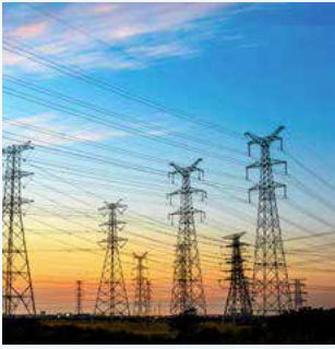
Power transmission towers
